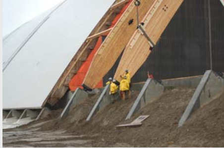
AGRIUM Potash Storage and Handling Vanscoy, Saskatchewan Structurlam Products
